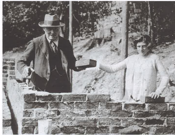
Winston Churchill and his daughter Sarah laying bricks at their house in Chartwell, Kent, September 1928
